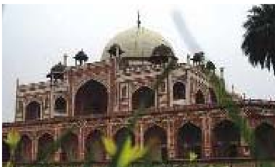
Restoration work at Humayun's Tomb, New Delhi facilitated by Aga Khan Foundation and the Aga Khan Trust for Culture
